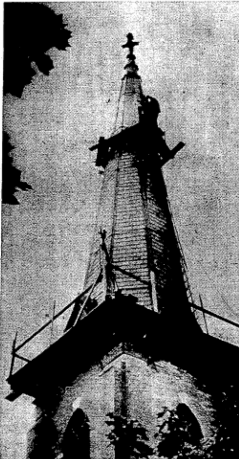
HIGH THERE —Motorists have been seeing some fancy footwork in the sky as workmen repair the steeple at Zion Evangelical Lutheran Church at Boulevard and McAdoo Avenue, Jersey City. (Van News Photo.)
